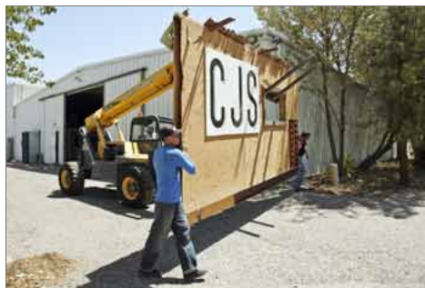
WORKERS MOVE A PANEL from a building Friday at CJS Studios in Avondale. The property was recently purchased by a developer who is going to have the studio destroyed to make apartments. Some of the Old West building façades will be preserved at Rawhide at Wild Horse Pass. View photo by Michael Clawson
